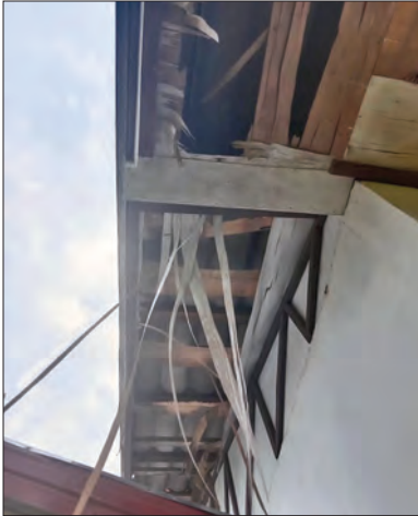
Eaves damage found at Ban Tha.
