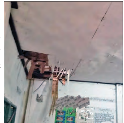
Ceiling damage found at Phon Thanh. There was very minor exterior damage.
