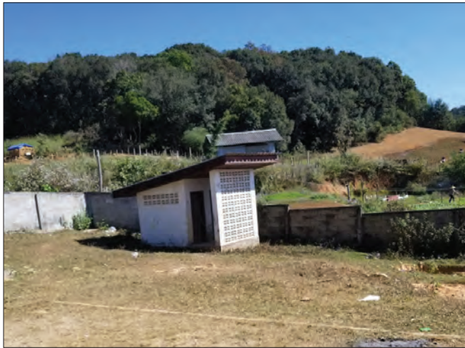
The old toilet at Yun Xay. The new one will be at a different location because this one floods during rainy season.
