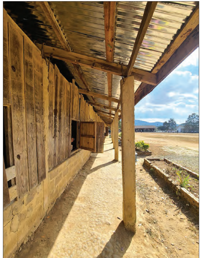
At Lat Huang High School, there is a new roof for which the TLC Brotherhood provided the materials. It appears they could use a concrete porch as well.
