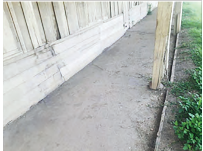
The "corridor" is dirt, which turns to mud in the rainy season. This project will provide concrete for the corridor and classrooms.
