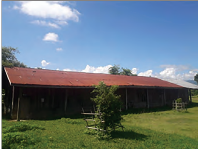
Rusty corrugated steel roofing is no longer doing its job and needs replacing. The request includes 460 of the heavy sheets, which villagers will install. Photos provided by local officials.
