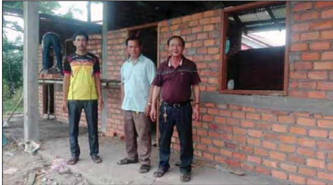
With other Lao officials, Ajarn Soundeuane, at right, visiting Ban Long Lan Pre-School construction.
