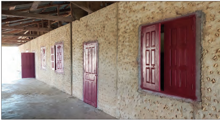
New doors and windows with new hardware and concrete repairs at Laht Saen Lower Secondary School, all thanks to TLC Brotherhood Assistance grants.
