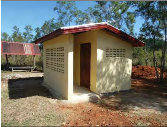
Ban NaFa villagers built this sanitary toilet using TLCB cement. A huge improvement over previous facilities that were in the way of a new road.
