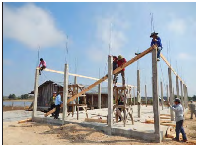
Ban Nong School construction underway in January, 2016. Local labor and wood, TLCB steel and cement. Photos by the author.
