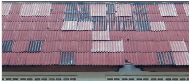
The first priority at Banteay Samre was the failing "holey" roof.
