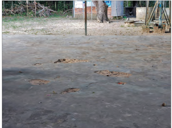
The original concrete floor at Banteay Samre Primary School was failing. Construction money came from outside, but there were no funds for upkeep. The villagers showed willingness to do the work.
