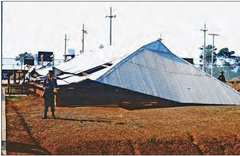
After passage of a "green monster" thunderstorm deep in the rainy monsoon season. This was once the 23rd TASS day room. Luckily no one was hurt in the collapse.
