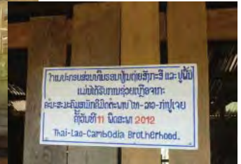
Above: this sign is typical of similar proclamations appearing in Lao communities we serve. My-uree Strouse kindly provided this translation: "The new tin roof and new floor were completed with donation from Thai-Lao-Cambodia Brotherhood Association, 11 May 2012."
