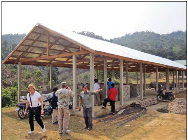
Below, 1a Khon Sana Primary School—This is the new building under construction. Nancy Sweet is in the foreground, and Mac is pointing something out to Roger Durant. This building will be a big improvement for the students at this school.
