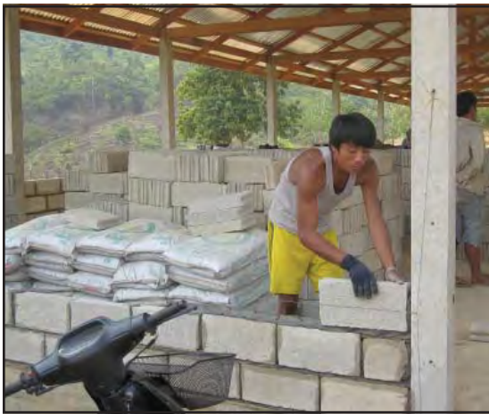
Above, Ta Khon Sana Primary School—The new wall is going up as we watch.
