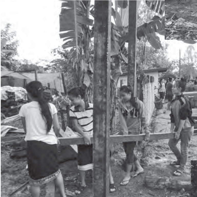
At left, girls carrying concrete fence posts, paid for by Air Commando Association funds through TLC Brotherhood. Above, boys placing posts around agricultural perimeter. Fence is used to keep feral pigs from eating the crops the children will raise. Below, PVC irrigation pipe used to connect concrete pipe sections used as sub-reservoirs in the fields. Water is pumped from the nearby river. Below left, school and Thakkek Province officials observe new water flow to fields.
