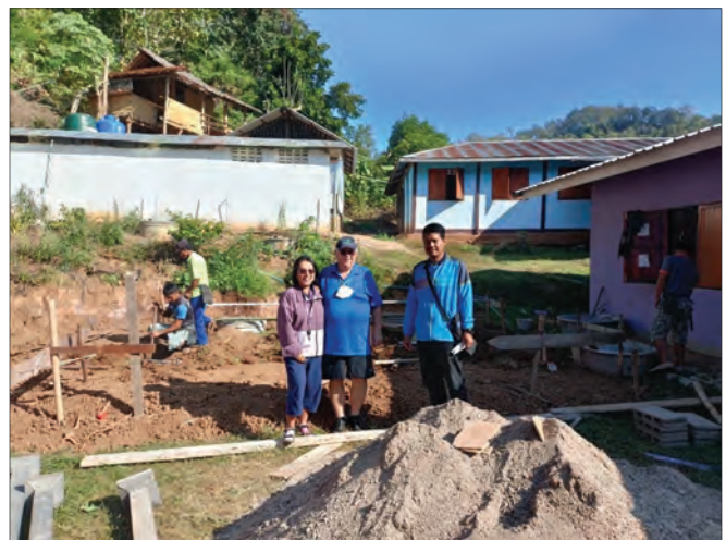
The start of the first new Assistance project in Thailand in quite a few years. Potjanee and Monty Dubs next to Principal Suwit of Ban Nam Phiang Din School. This plot will be the site of a new bathroom. Photos provided by Principal Suwit to Monty Dubs.
