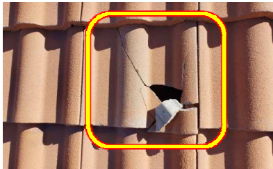
Damaged roofing tiles
