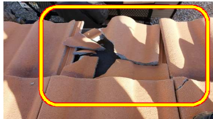
Damaged roofing tiles
