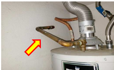
TPR pipe runs uphill
