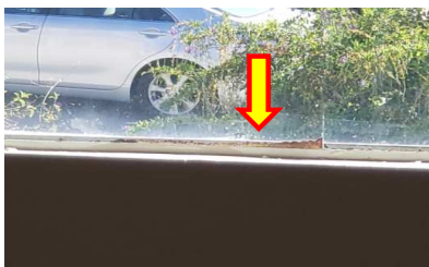
Damage between glass
