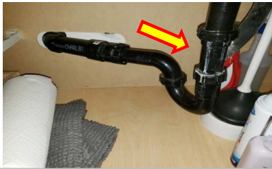
Sink drain leak
