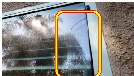
Broken glass pane
