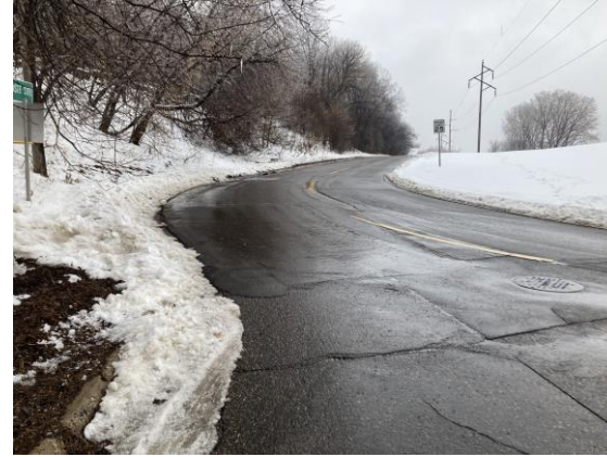
Springs/seeps along Linwood Park requires frequent maintenance in winter with ice build up
