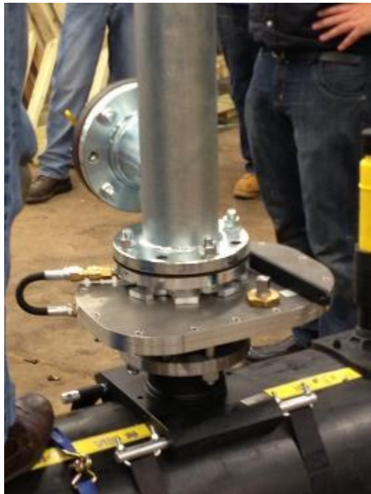
Figure 8. Kleiss BZA-4-G2 system attached to an electrofusion fitting on an 18” dia. PE pipe
