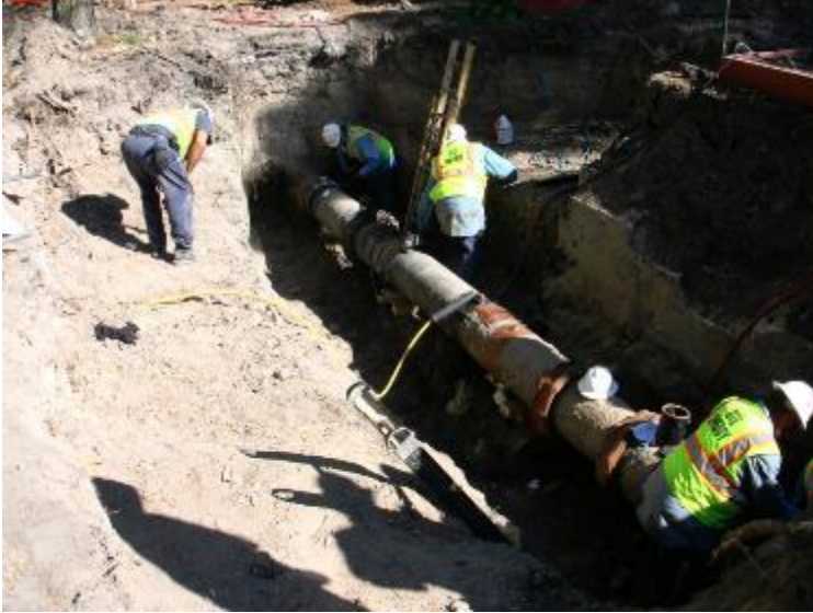
Figure 35. Michigan Gas Utility 16” cast iron main
