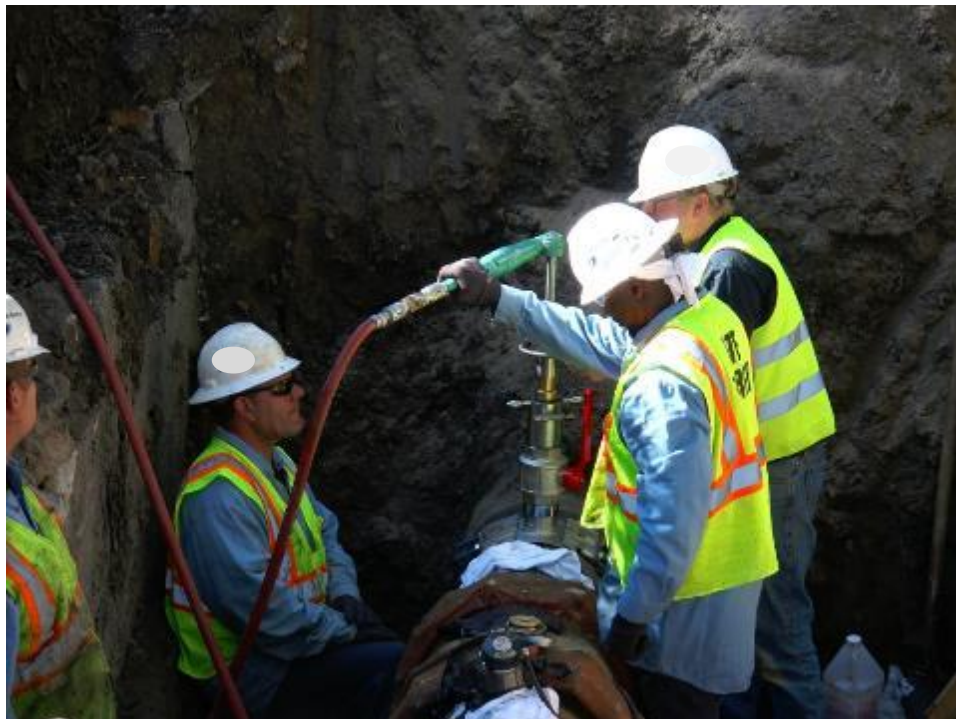
Figure 38. Michigan Gas Utility crews tapping the 16" cast iron main using the Kleiss equipment
