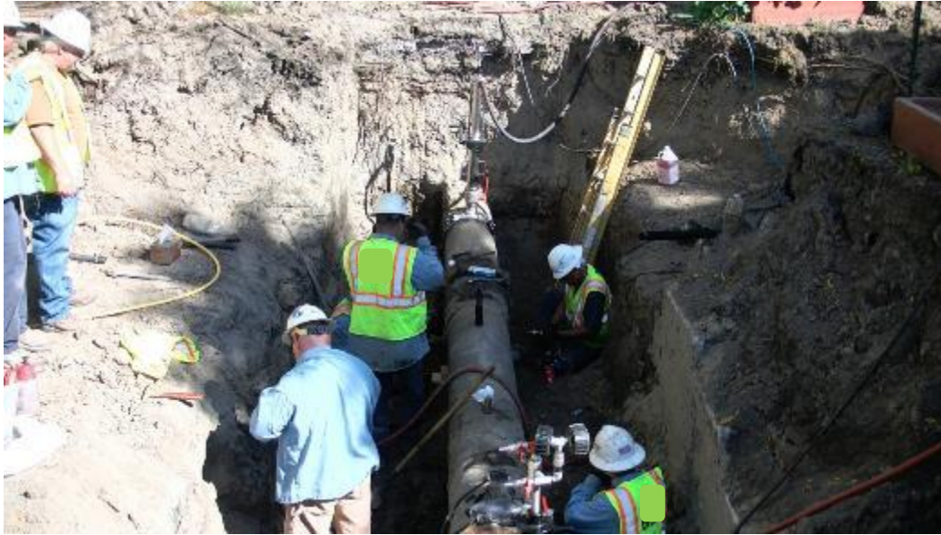
Figure 41. Michigan Gas Utility crews removing the drip pipe with the 2 Kleiss stoppers installed
