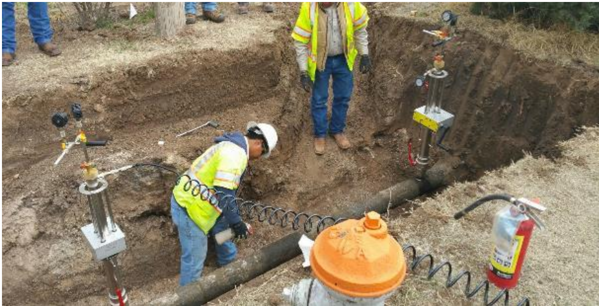
Figure 52. Kleiss field demo at Gas Utility #4
