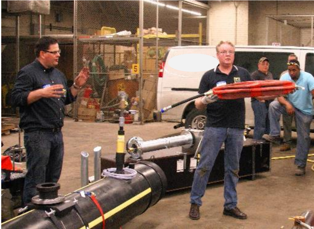
Figure 43. Kleiss bag used to stop off the flow in the 18” PE pipe and EF fitting on the 18” pipe
