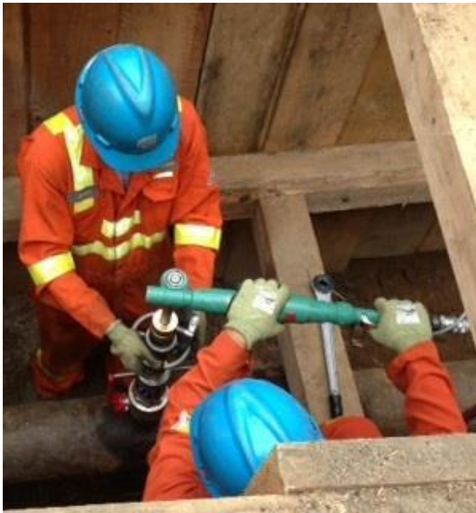
Figure 49. Gas Utility #3 crews using the Kleiss equipment to tap the 8” steel pipe
