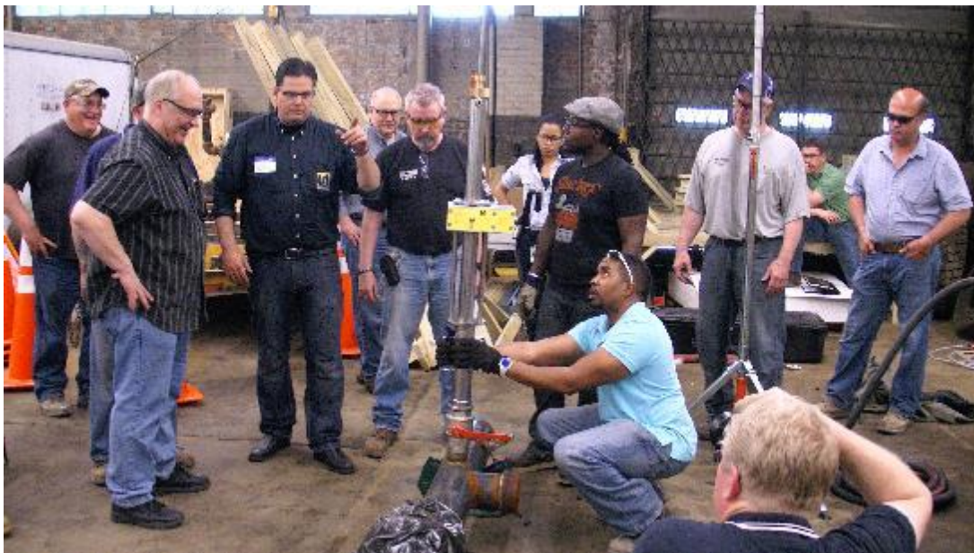
Figure 46. Gas Utility #2 personnel installing the Kleiss BZA-4-G1 stopping equipment on a 6-inch steel pipe
