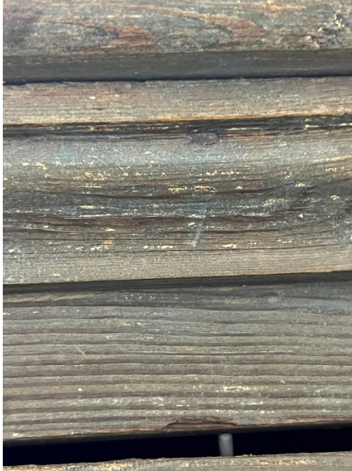
Figure 23: This photo shows one of the smaller nails attaching the top molding. It is so well placed it is barely visible, top center right.
