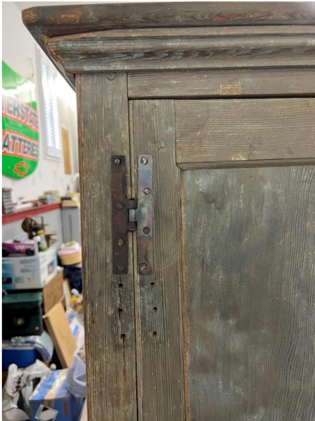
Figure 5: This photo shows the original hinge after being repaired by master blacksmith Alex O’Dell of Orange, Virginia.
