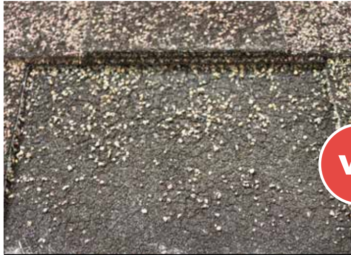
Standard Asphalt Roof With Severe Granule Loss
