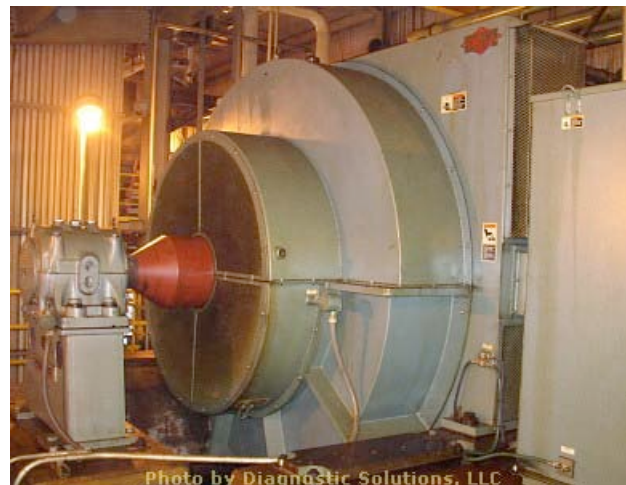
Figure 7.8 Synchronous 3850-hp Motor
