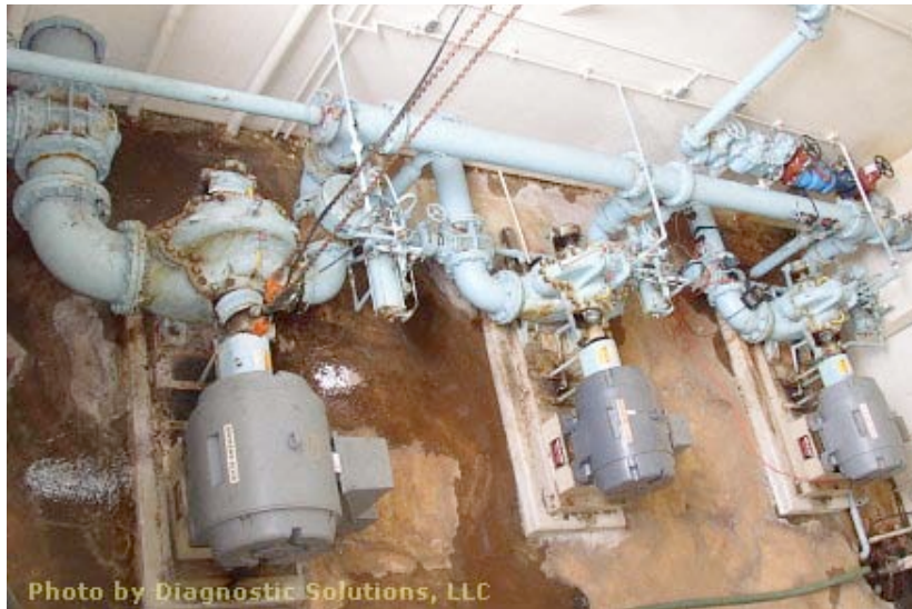
Figure 7.13 Pumping system layout with poor suction geometry (and little opportunity for improvement)
