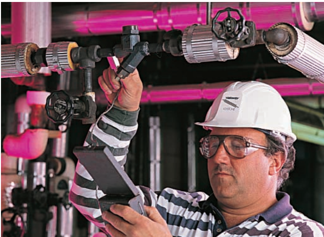
Fig. 6—This operator is using a contact pyrometer to make upstream and downstream temperature measurements to determine trap performance in a closed condensate return system.
