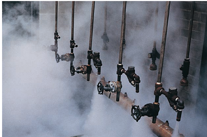
Fig. 5—Determining trap performance by the sound method is difficult where many traps discharge in close proximity. Temperature measurement method is preferable.
