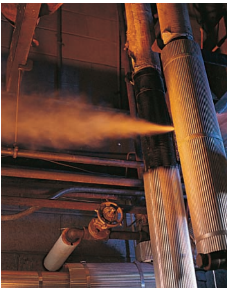
Fig. 1—Ruptured tracing is a typical and costly steam loss.
