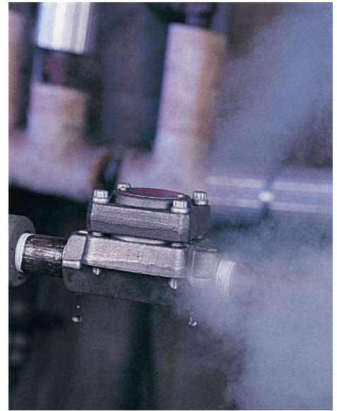
Fig. 2—Defective gasket of this trap permits loss of live steam from the system.
