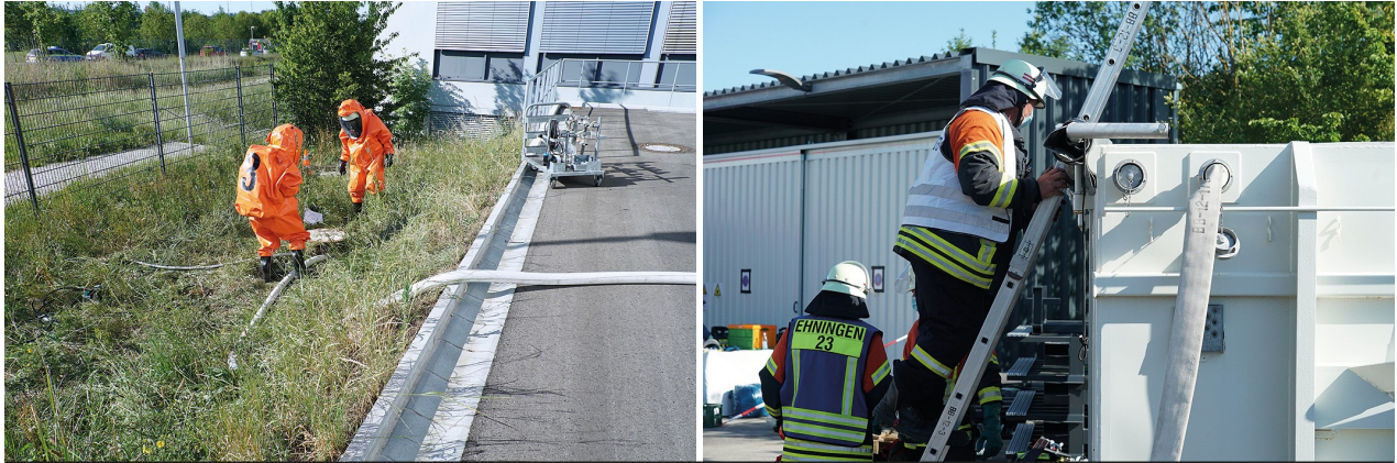
Left: The extinguishing agent mixture was first collected in the underground structural five-cubic-metre collection tank ... right: ...and then pumped into the company's liquid-tight roll-off container (here during preparation for the pumping work).
