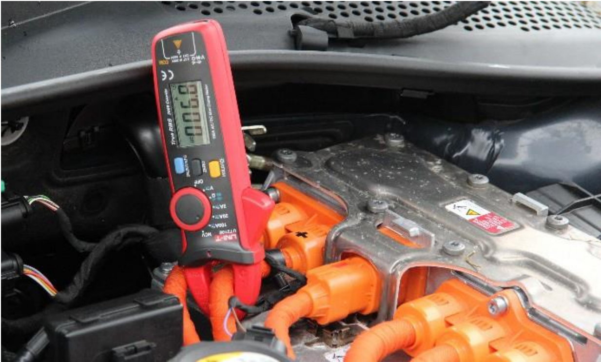
Figure 49. Inductive ammeter clamp on a high voltage cable (measuring the current drawn by the EV cabin heater)
