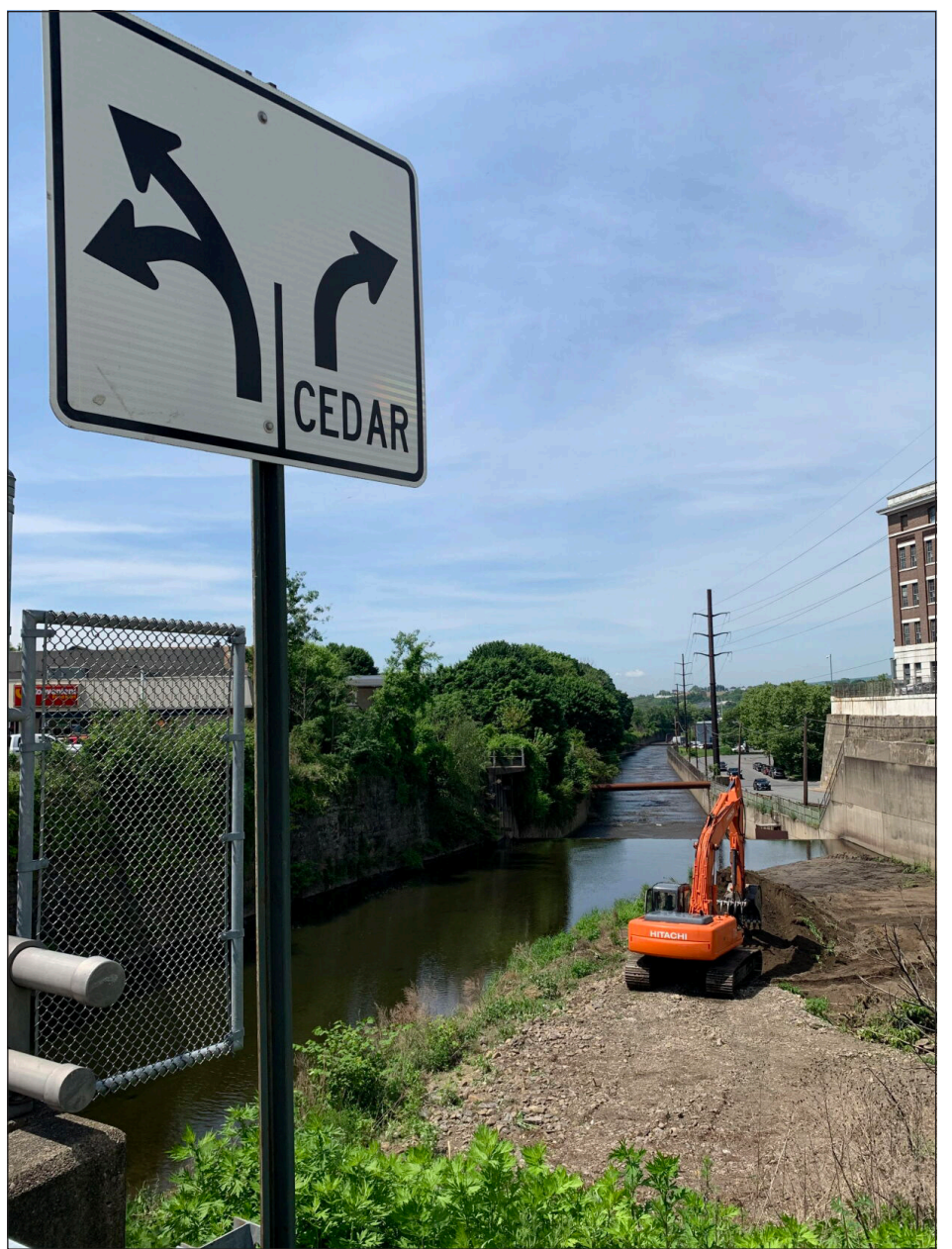
A contractor for the city Scranton on May 20 does sediment removal and stream restoration work in Roaring Brook near Cedar and Mattes avenues related to a 2018 storm flooding declaration under the Federal Emergency Management Agency, city officials said. JIM LOCKWOOD/STAFF PHOTO
