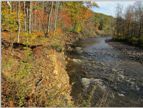
Erosion highwall cut at Chicos Bend in Cobb's Gap
