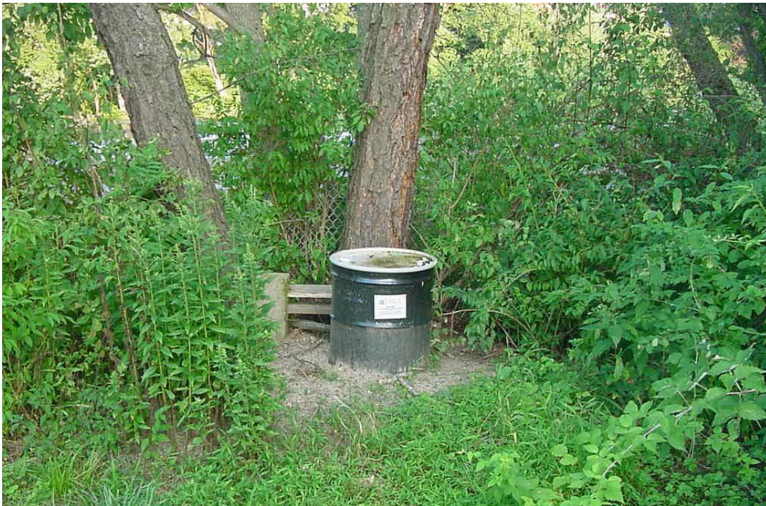
Figure 6-5 Metal drum anchored in concrete on the riverbank containing transducer hookup.
