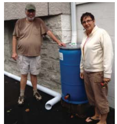
Downspout disconnect with rainbarrel.
