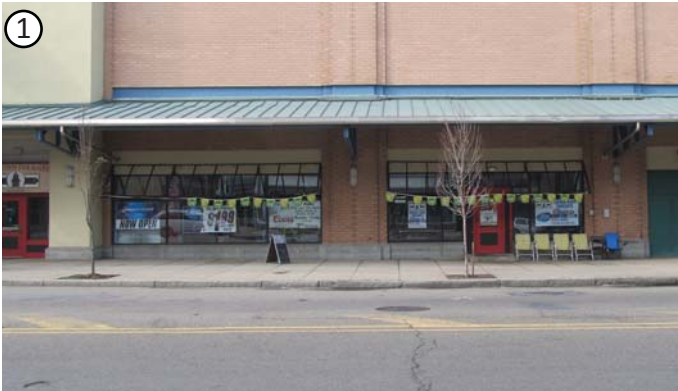
Stretching along Lackawanna Avenue are a series of overhangs that direct stormwater into the building through gutters.
