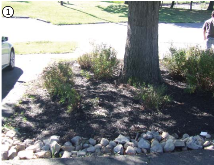
1 A small rain garden has been installed in an existing gap in the parking lot.
