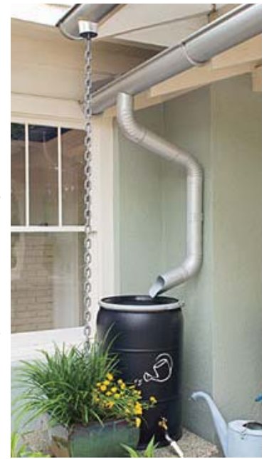
A downspout being directed into a rainbarrel.
