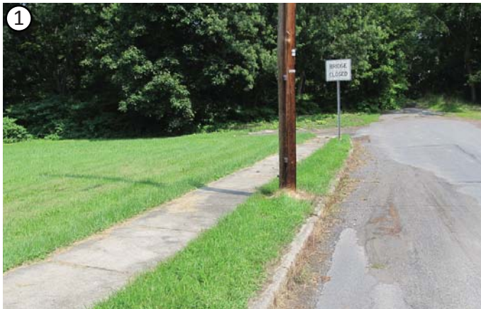
Water currently runs along the existing curb and into Leggett’s Creek at the end of the road. In this picture, the transported and deposited sediment is visible.
