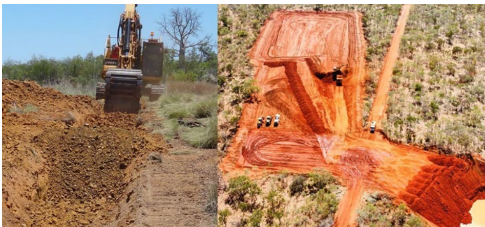
Figure 4: Bulk sampling of shallow gravel. Figure 5: Mining & backfilling in the L Channel.
