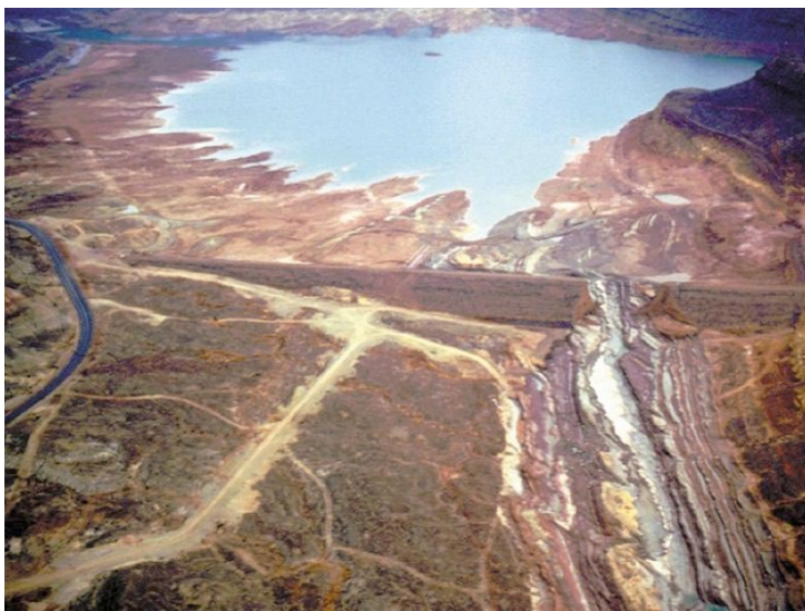
Quail Creek Dike Shortly After the Failure Photo Source: Utah Geological Survey
