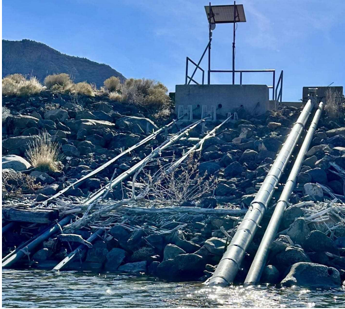
Photo No. 2 shows the north face of Gunlock dam. If it were located in Ivins, we would call it urban industrial blight.
