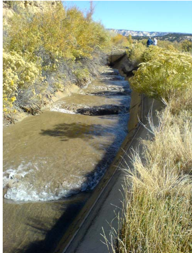
Wide Hollow sedimentation basin with accumulated sediment. (Photo courtesy Franson Engineering)
