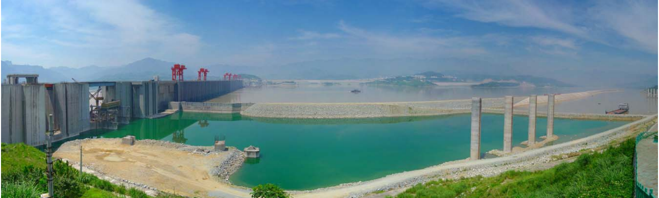
Three Gorges Dam under construction near Sandouping, China, 2004. Sediment management techniques employed at the dam will be among the most sophisticated anywhere in the world. (Photo permission by Wikipedia Commons License: http://commons.wikimedia.org/wiki/Commons:GNU_Free_Documentation_License )
