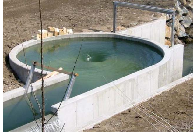
Example of a vortex installed in a conduit to remove sediment. (Photo courtesy of Sepp Hasslberger.)
