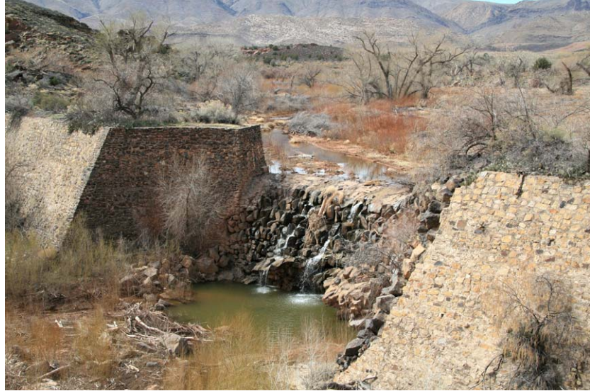
Winsor Dam, downstream of Gunlock Reservoir on the Santa Clara River, diverted water for the Ivins Canal and Reservoir. Built in 1933, the impoundment has entirely filled with sediment.
