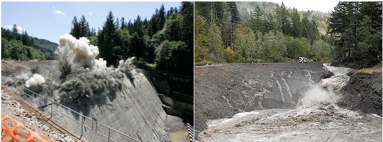
Demolition of Marmot Dam and subsequent erosion of sediment deposits behind the dam. Cherryville, Oregon (Photos courtesy of Portland General Electric.)
