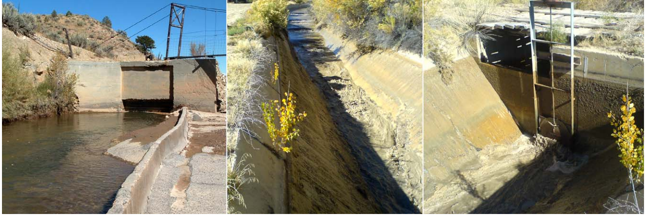
Left: Entire flow of Escalante River being diverted into the inlet canal to Wide Hollow Reservoir. Note sediment. Middle: Sediment being flushed from the sediment basin in the enlarged canal. Right: Sediment leaving the sediment basin through the downstream sluice gate at a right angle to the basin. Flow and sediment return to the Escalante River. Also see the upper left photo on the cover of this report. (Photos courtesy of Franson Civil Engineers.)
