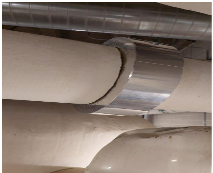
NAWT Collar installed on Cold supply to Domestic Hot Water Heater
