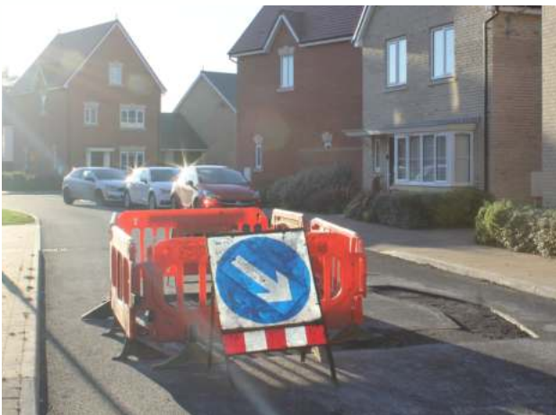
Damaged road and over-reliance on on-road parking - it is important that new construction is undertaken to a very high standard so that roads and buildings are long-lasting and the need for premature repairs (which affect residents' quality of life and increase the embodied carbon associated with a scheme) is avoided
