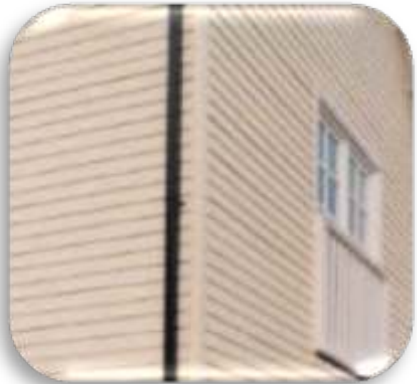
Inappropriate "Shiplap" weatherboarding
