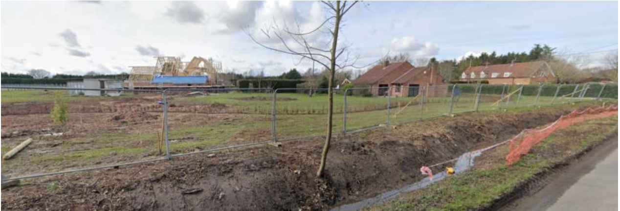
Dwelling under construction at Pond House - view from Coggeshall Road c. March 2021
