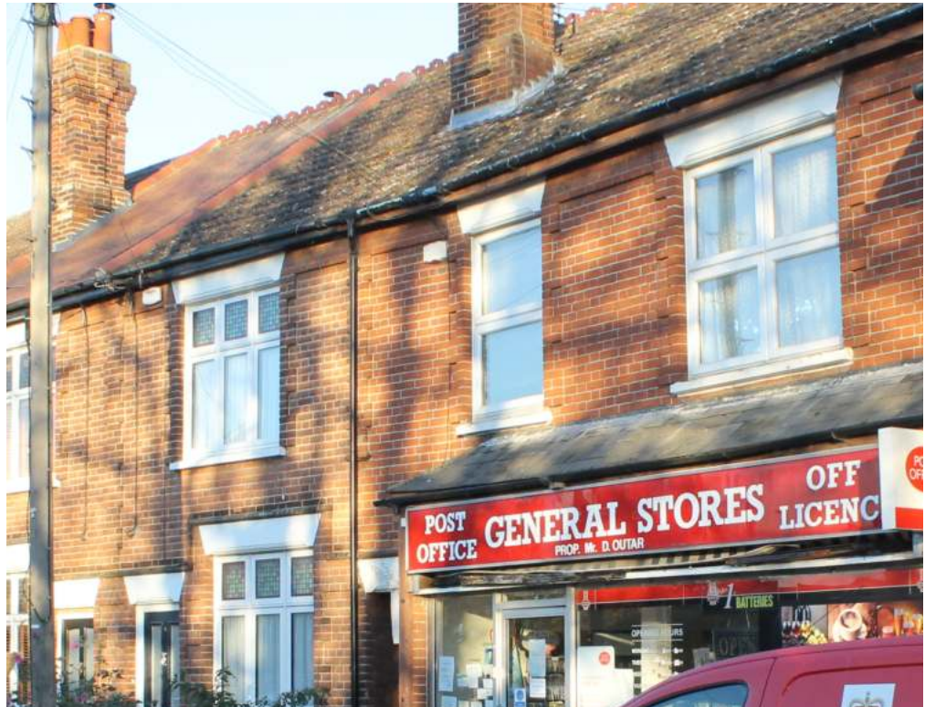
The loss of some of Khartoum Villa's original timber windows (featuring beautiful leaded light transoms) is unfortunate and detracts from the character of the whole terrace
