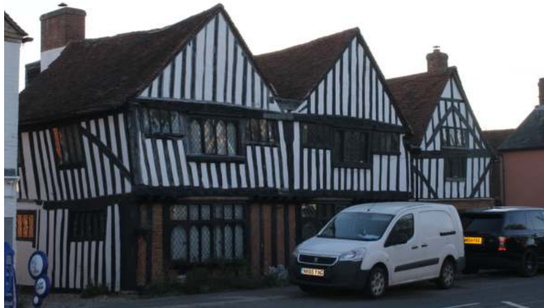
Repair work sensitively undertaken at Ancient House, including repair of roof, gutters, flashings and chimneys
