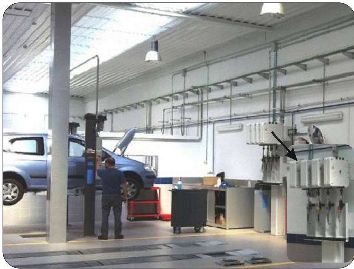
Oil Dispensing Gun with Hose installed at Two Post Lift Area
