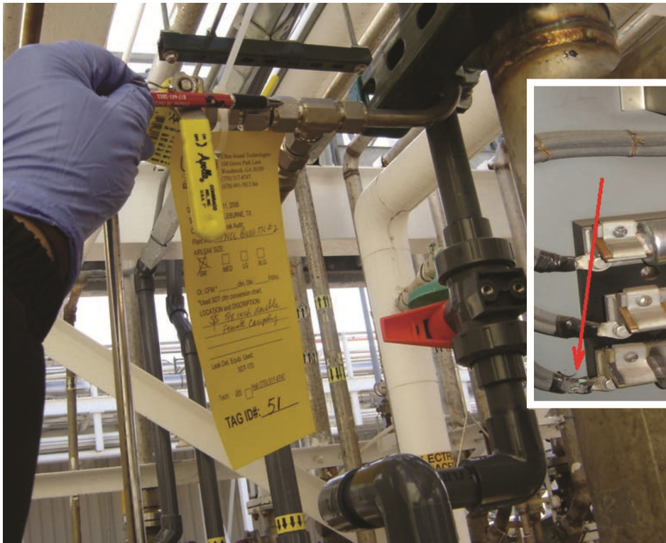
Figure 1: Air leak audit, chemical plant, Waco, TX
