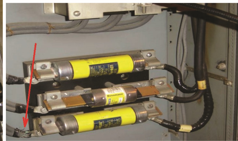
Figure 2: Electrical arcing heard within closed 480v panel at a power generation plant
