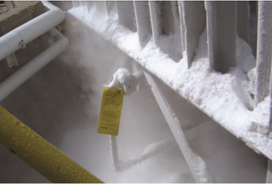
Figure 4: Leak on a liquid oxygen supply system
