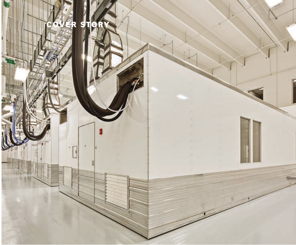
Each G-CON POD is served by its own independently controlled, redundant HVAC system.
