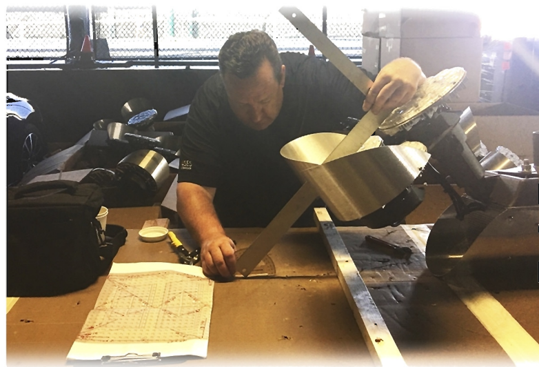
Nelson Scott, COO & Founding Owner took a hands on approach in making sure the fixtures were angled correctly to achieve the precise and correct light distribution for the California Tennis Club
