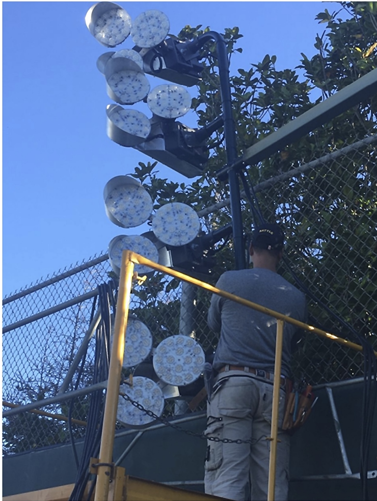
Erwin Dimacali modified the Cal Club's fixture heads to accept additional LED fixture heads a key component in achieving a successful outcome in this sports lighting project
