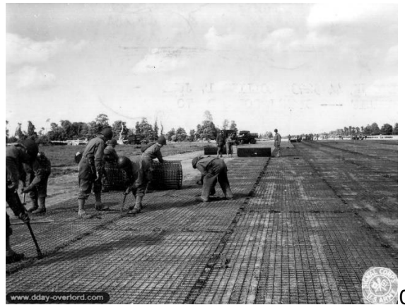
Square Mesh Tracking Runway being laid at A-6 Beuzeville au Plain, June 1944 Picture from US National Archives
