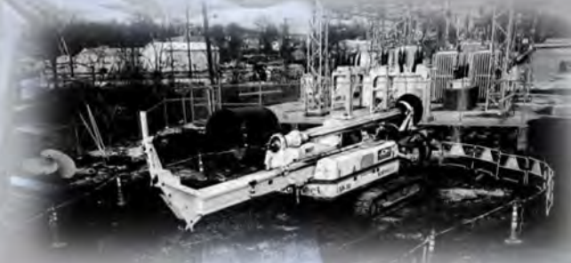
Typical set up of both Hard & Soft Barricades to prevent unauthorized entry Duke Energy Brazil
