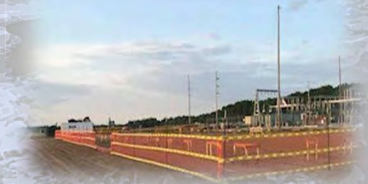
Temporary caution fence installed to control work area access entry at an existing AEP owned substation located near South Bend IN
