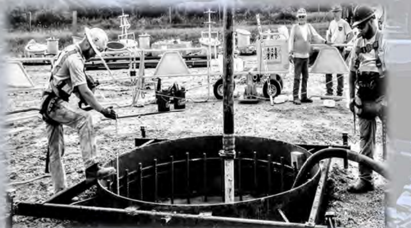
Above: Men maintaining 100% fall protection while pumping concrete for a 8'x 47' Drilled Shaft AEP Ohio
