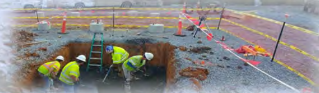
Barricade Fencing & Proper Egress being utilized at a Substation under constructio for AEP in TN
