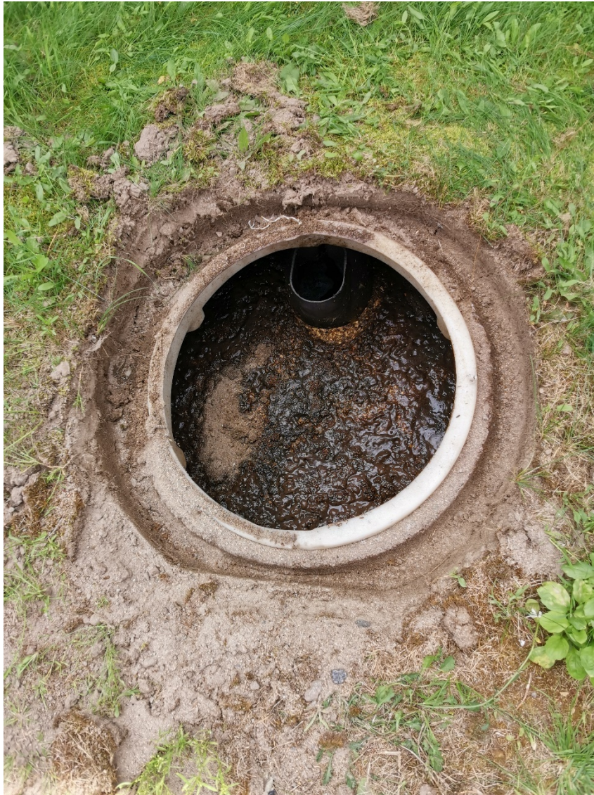
Figure 2: Inlet Chamber of the septic tank (Working level – 3.5 feet – sludge measurement 4 inches, scum measurement 1-1/8 inches)
