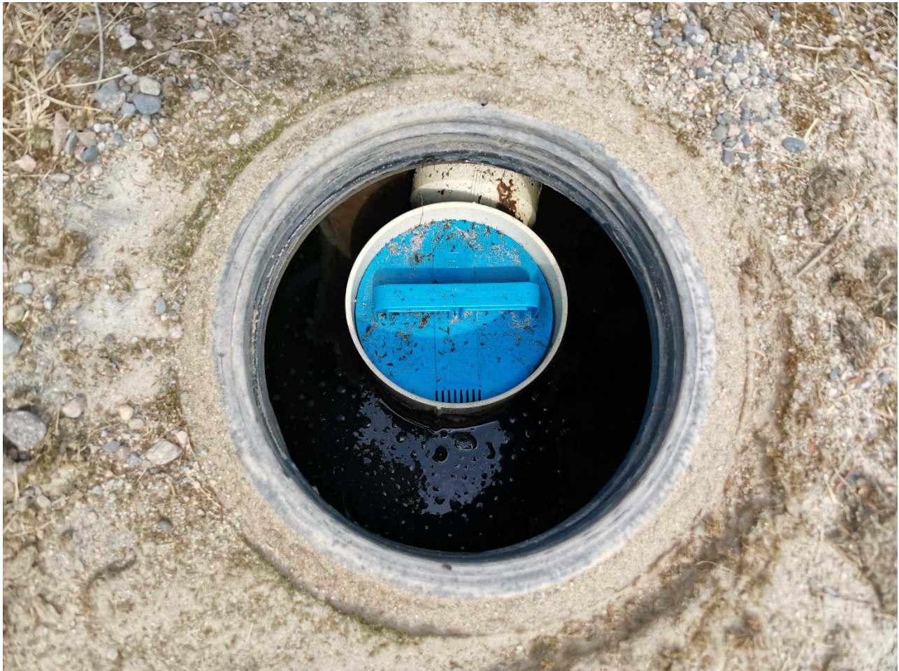
Figure 3: Outlet Chamber of the septic tank (Working level 3.5 feet, sludge measurement < 1 inch, scum measurement < 1/8 inch)
