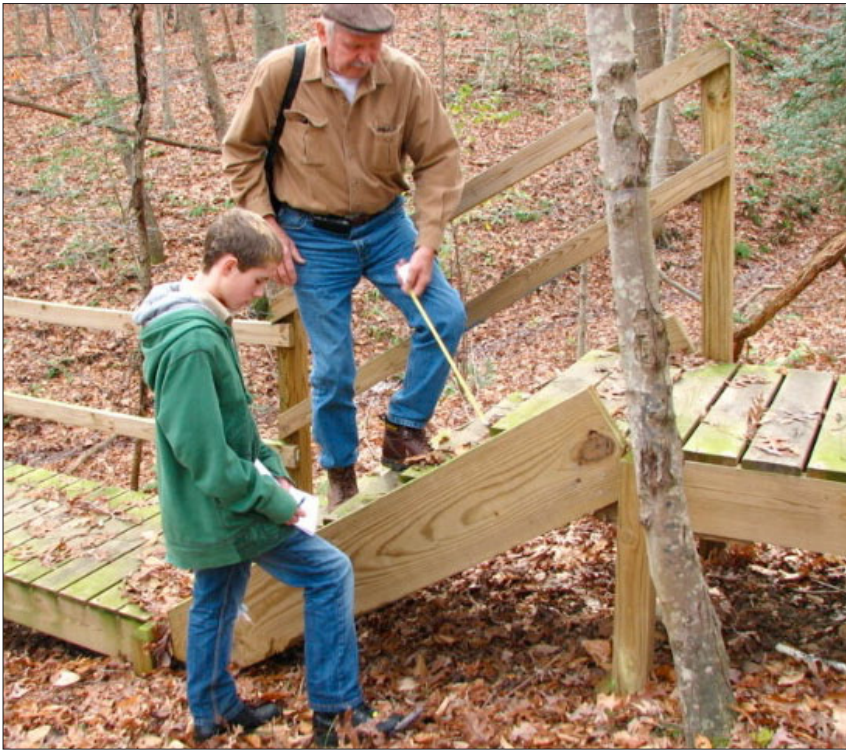
Scout Brian Stroh is in the planning stage to replace a bridge for earning his Eagle Scout Badge. He recently visited the site where he took pictures and measurements. Photo by Kate Stroh.
