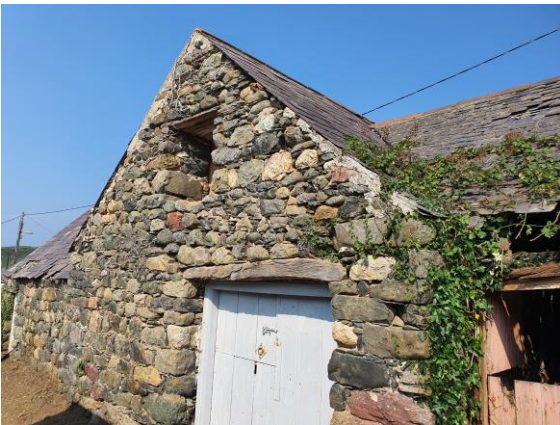
Gable wall of the south eastern end of the Mill Range with the Grain Dryer (left) and Stable (right).
