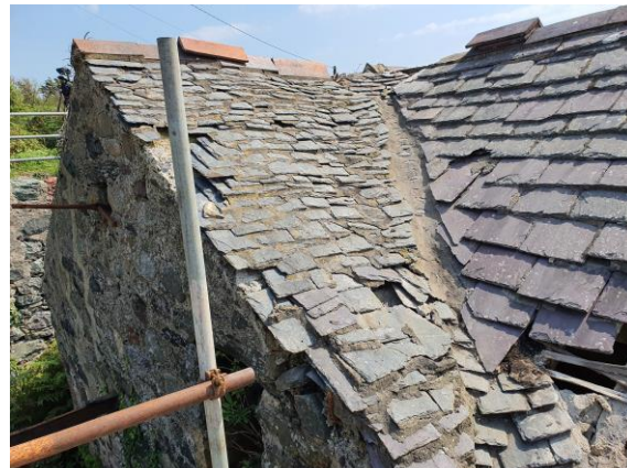
Welsh valley with random diminishing slate roofs of the Dresser Range and north gable of the Mill Range.
