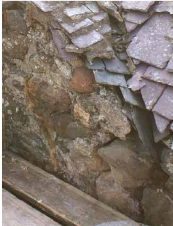
Figure 10, The eave of the Welsh valley appears to have had little overhang. Consequently, the masonry mortar below has been washed out.
