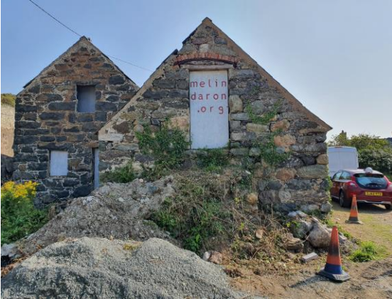
Front elevation with the gable walls of the Grain Dryer (right) and Dresser Range (left).
