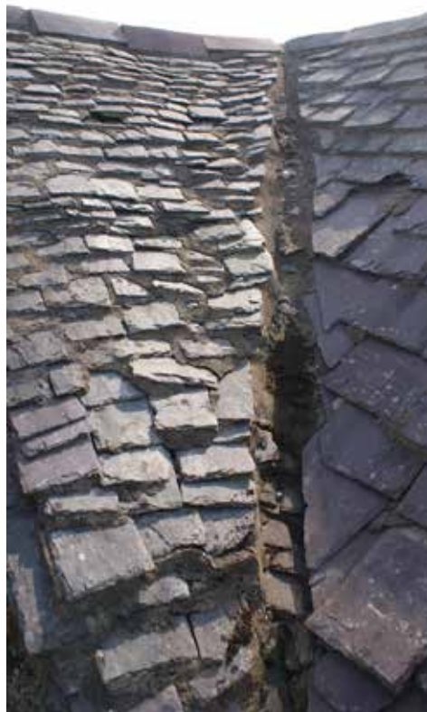
Figure 2. Area 2. The earliest Ordovician age slating from the Blaenau Ffestiniog to Cricieth area. Small random sized slates and the Welsh valley showing the mortar in-fill which is partially removed in the lower section
