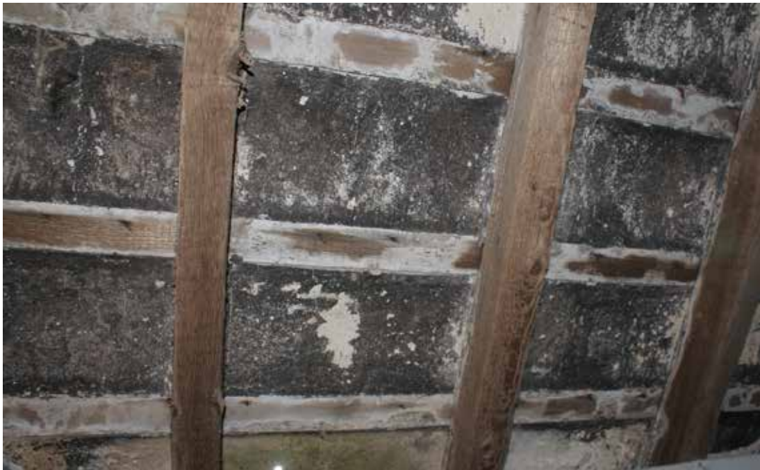
Figure 6. Area 5 Centre-nailed slating on sawn laths and torching. The slate nails are visible in the laths
