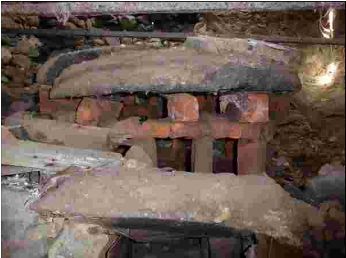
Plate 42: Perforated stack behind the firebox
