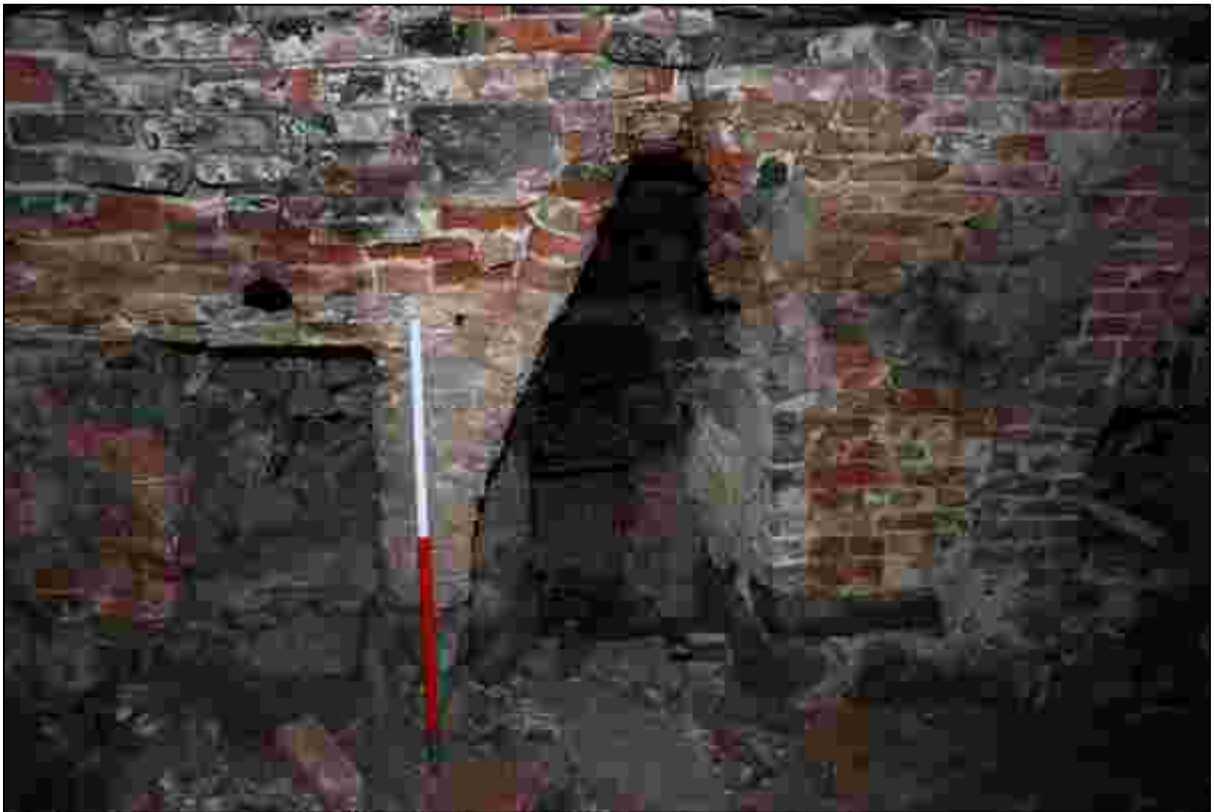
Plate 36: The northern and central opening in the dividing wall of the corn dryer
