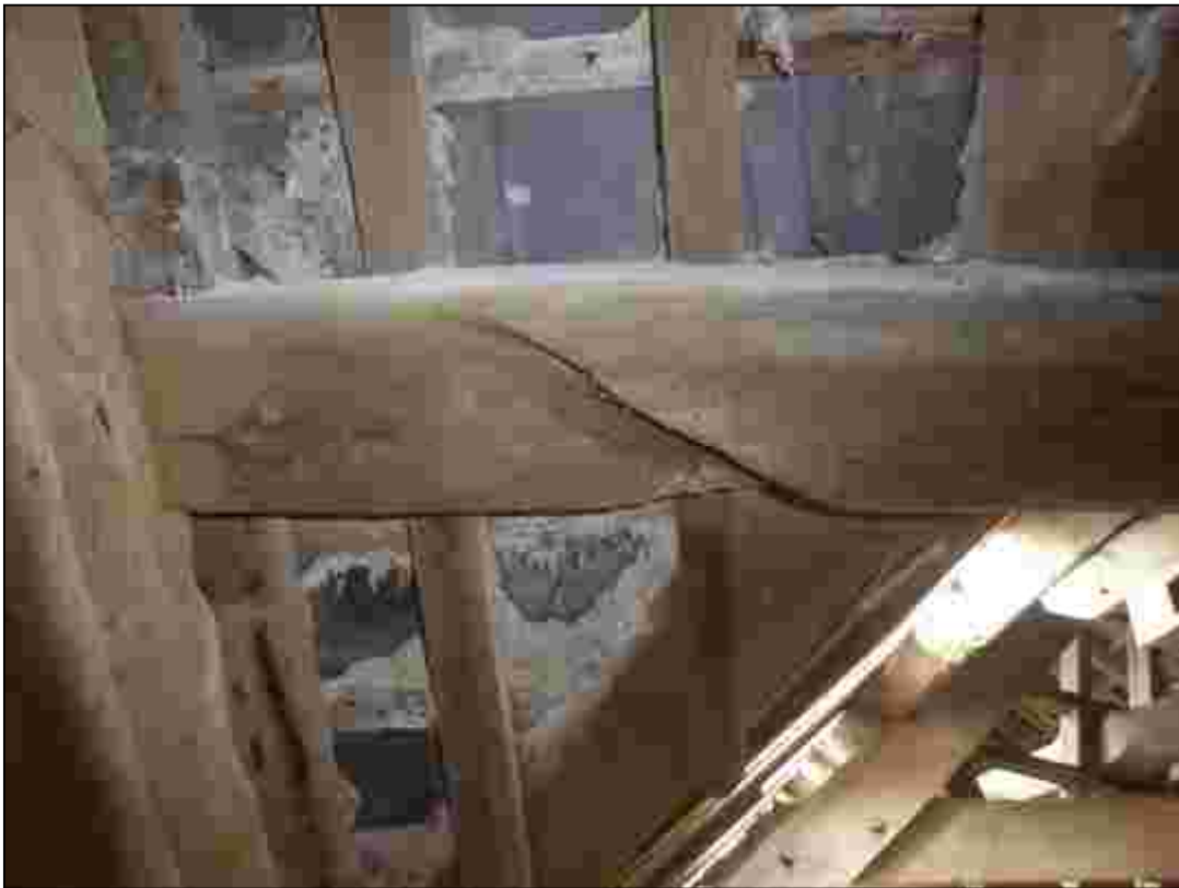
Plate 28: Worn slot in the purlin
