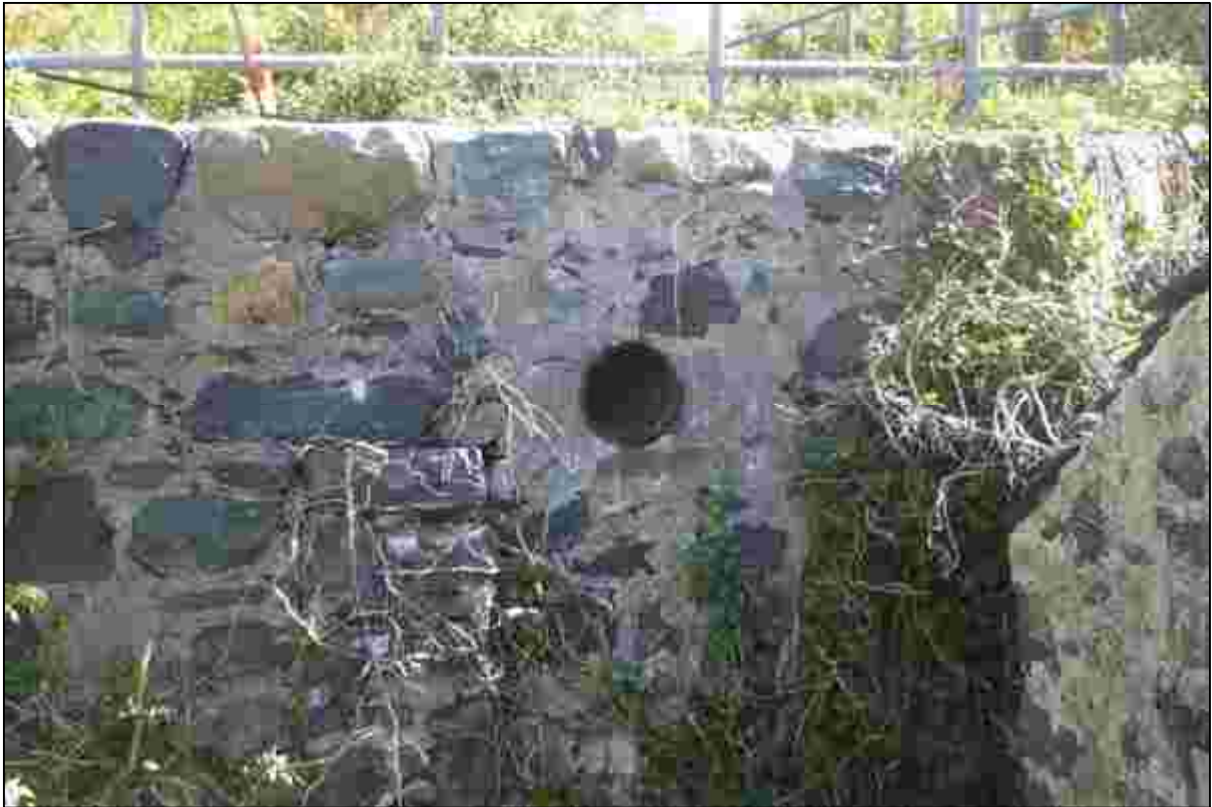
Plate 3: The outfall pipe and position of the launder
