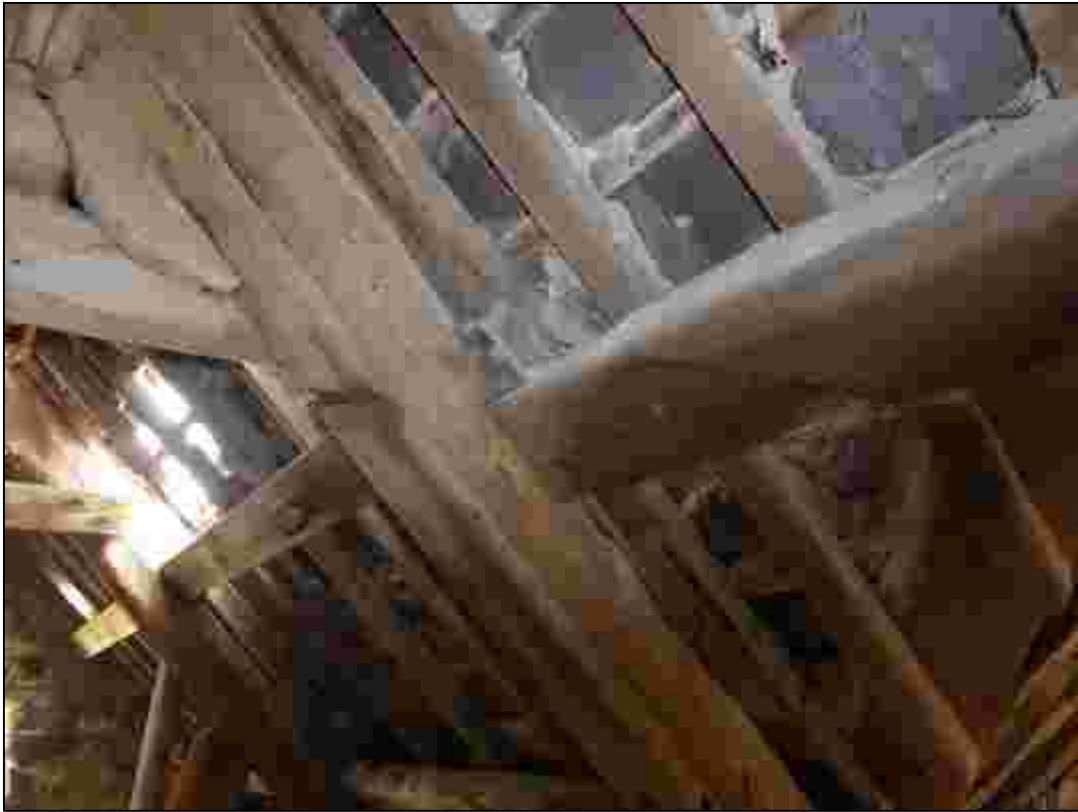
Plate 27: Worn slots on Truss 2 and its associated purlin
