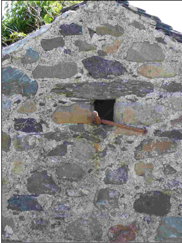
Plate 9: Opening for the control of the penstock
