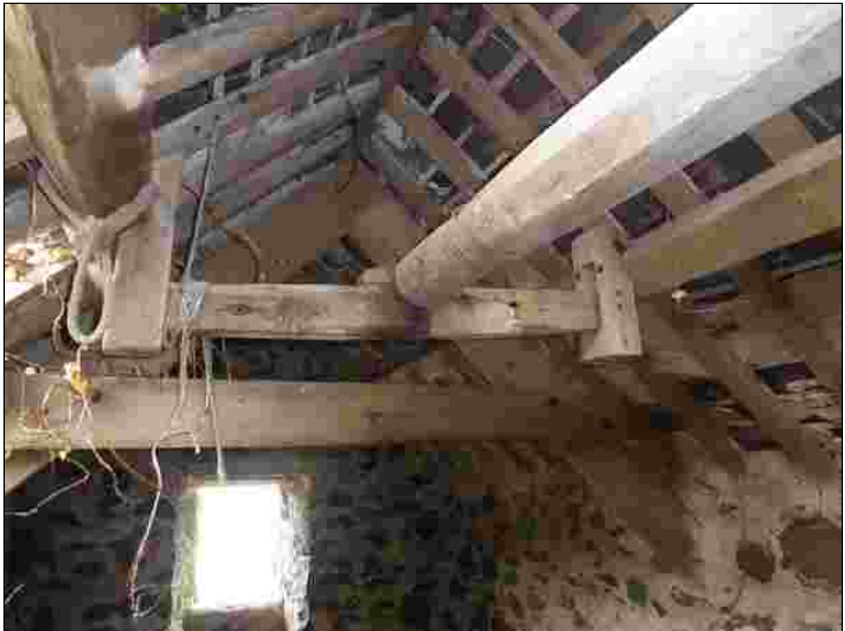
Plate 98: The worn section of the upper lay shaft above the hatch
