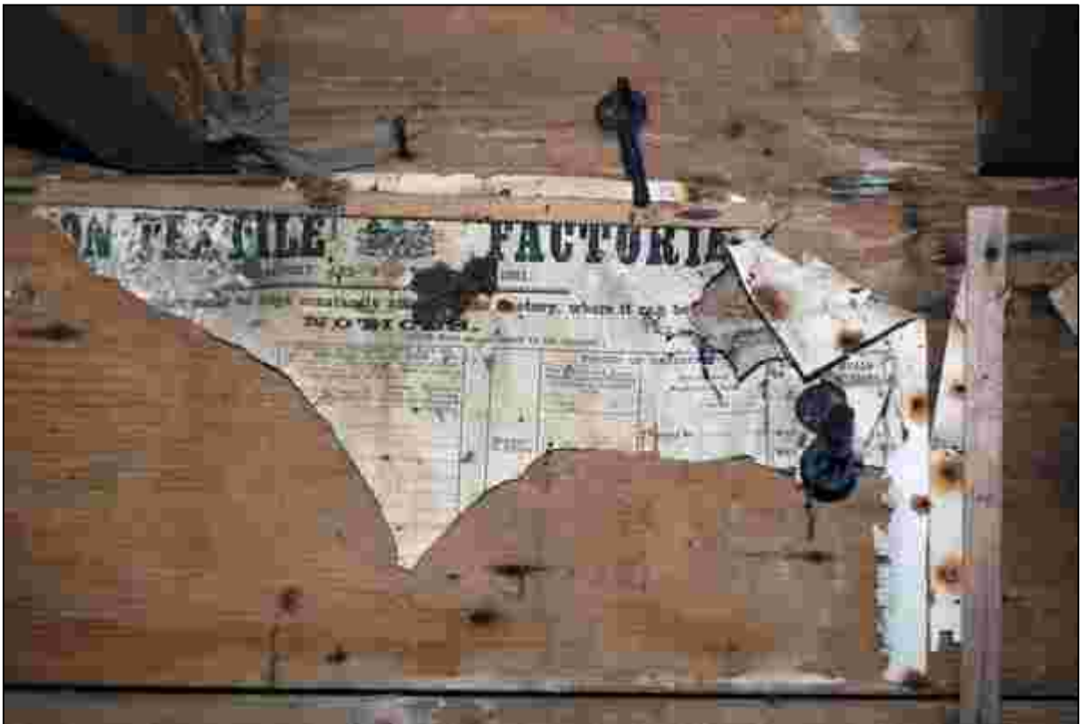
Plate 106: 1901 Factory and Works Act record
