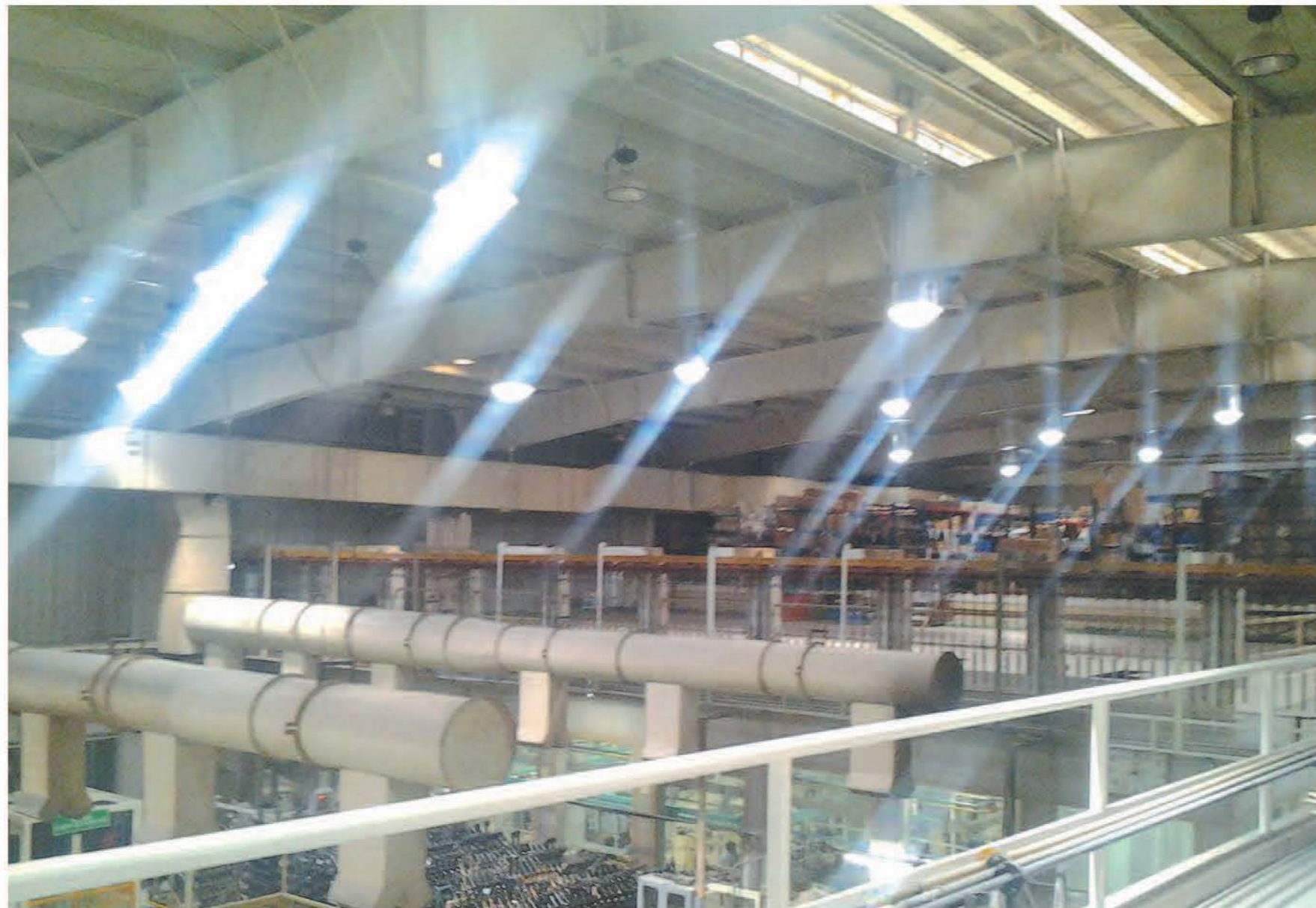
The image depicts an iEHS initiative, at one of the Anand facilities, to capture daylight
