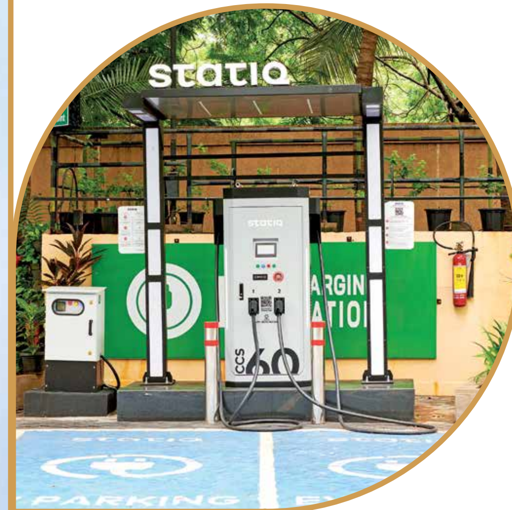
EV charging station – ITC Grand Chola
