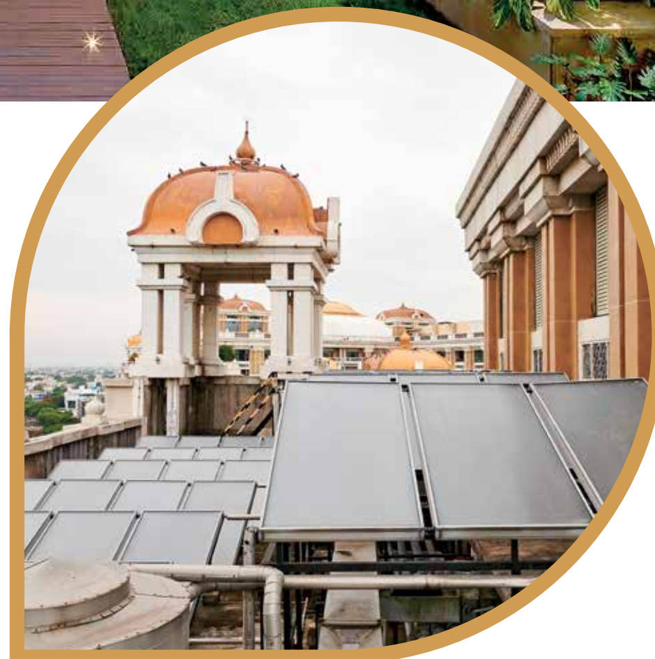
Solar panels - ITC Grand Chola
