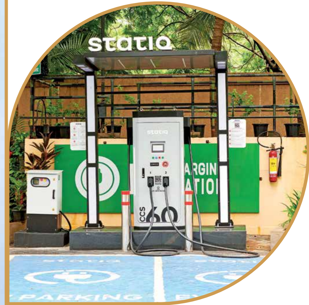
EV charging station - ITC Grand Chola
