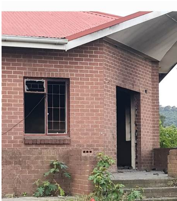
Delapidated former structure
