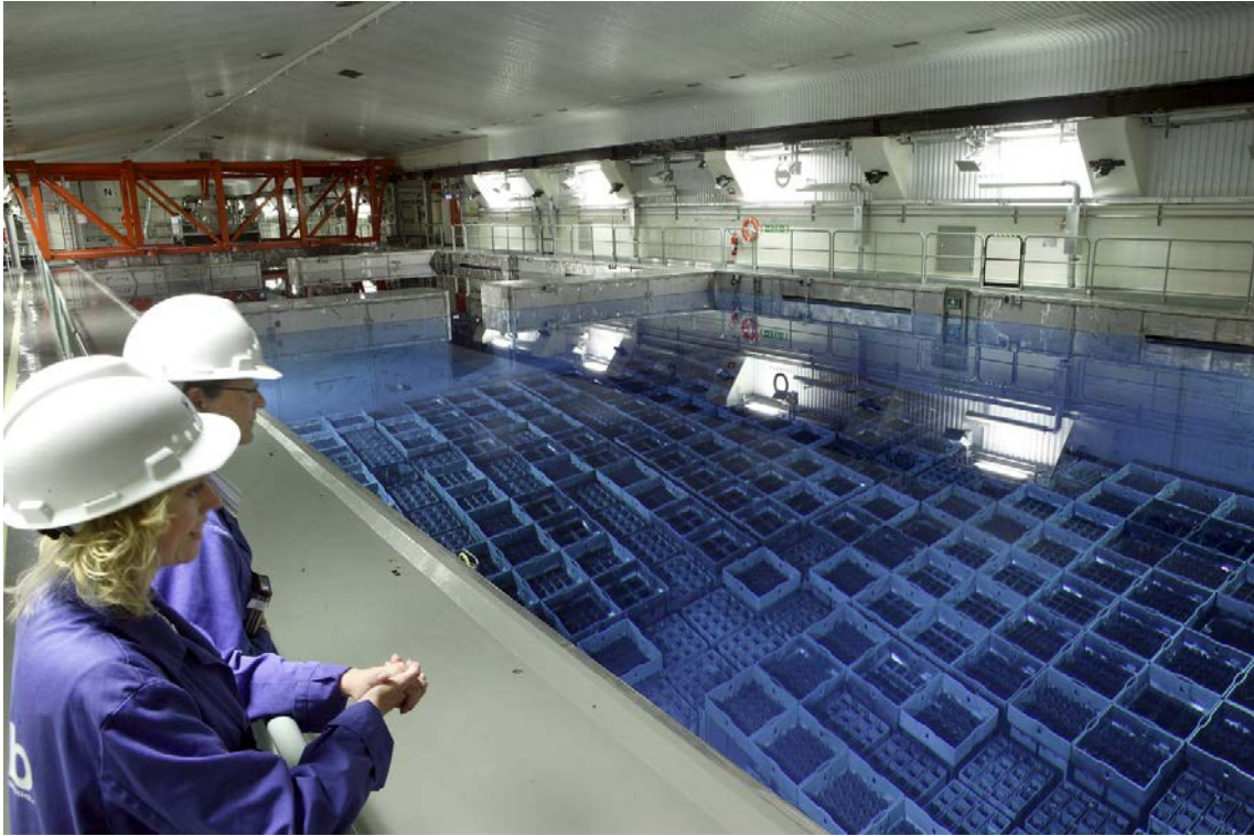
FIG. 7. The interim storage of spent fuel at Clab, Sweden (courtesy of SKB).
