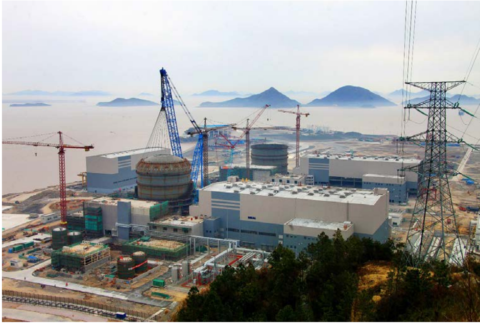
FIG. 3. Construction of the Sanmen nuclear power station, China (courtesy of China National Nuclear Corporation).
