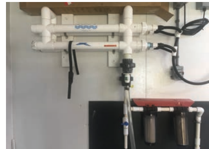
▶ Seawater filter and UV-sterilization system.
