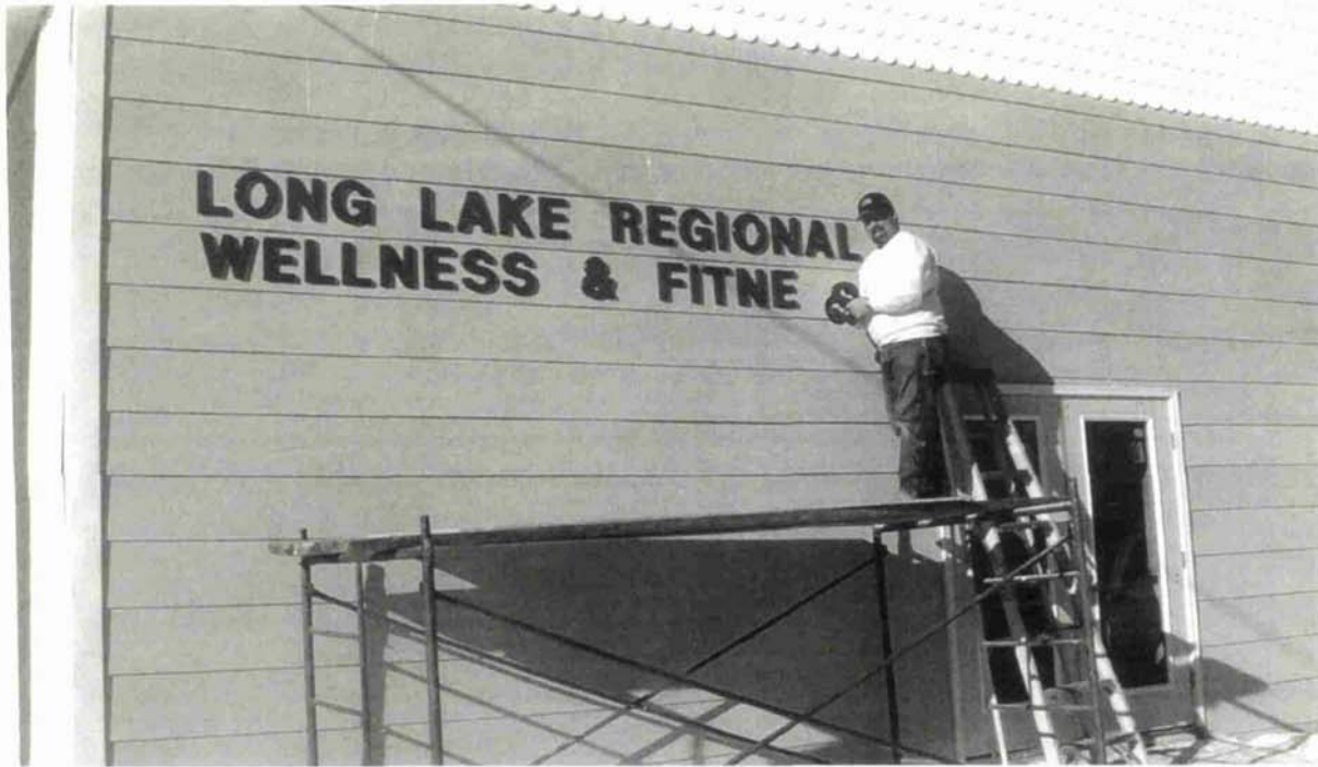
The center, owned by the Town of St. Agatha, is located at the Knights of Columbus Hall complex at 413 Main Street. The center open its doors to the public March 8, 2007. Installing the letters on the building - Dale Sirois.
