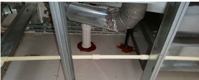
Fire-rated wall and floor systems are defeated if joints and penetrations allow fire and combustible gasses to make "end runs" around rated systems and assemblies. Every building trade is responsible for installing firestop associated with their work.
