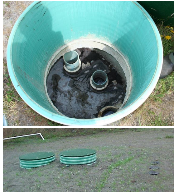
P-6.3: Influent Flow Tank
