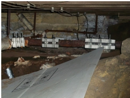
Bandaidd Steam Pipes
